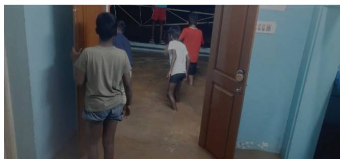
Storm water floods Holy Cross School
